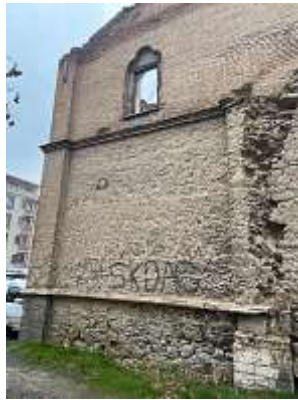
Figure 17: Vandalism on Armenian Protestant Church Walls (Source: Author’s Archive, 10.11.2021)
